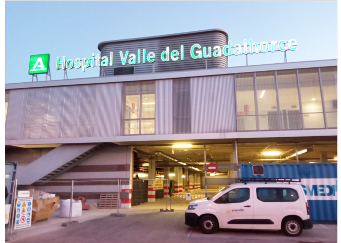
Valle del Guadalhorce Hospital, in Cártama, Málaga Consultant: EDAM CAD Services Commercial Building
